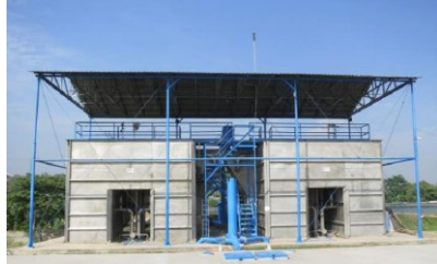
Pengolahan Air Bersih Water Treatment Plan
